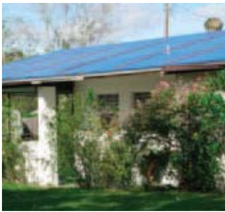
A hurricane-damaged roof in Orlando is temporarily repaired with a blue "FEMA tarp" provided by the Federal Emergency Management Agency.
